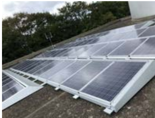
12 kw for generation
